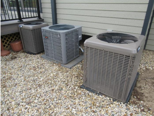
Exterior condensing units at clubhouse
