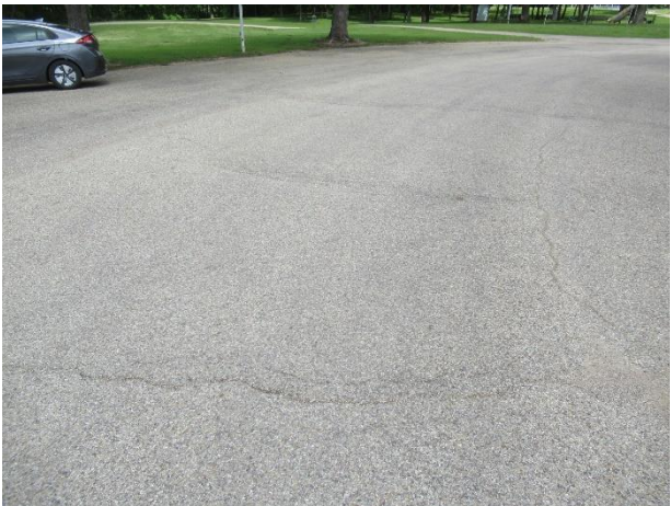
Pavement cracks visible throughout clubhouse parking area
