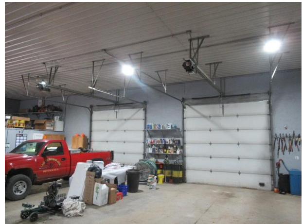
Overhead doors and operators
