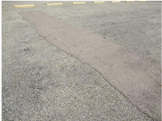
Pavement patch at beach parking area
