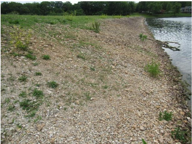
Rip-rap erosion at front face of the dam
