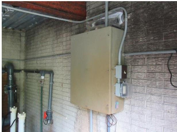
Pool equipment electrical panel
