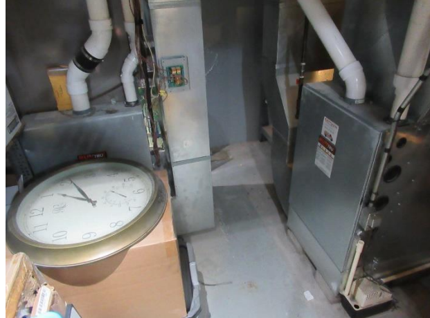
Interior forced air furnaces at clubhouse
