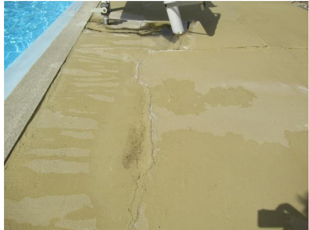
Concrete cracks at deck
