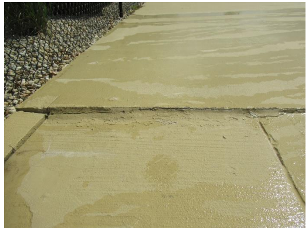
Isolated trip hazard at control joint
