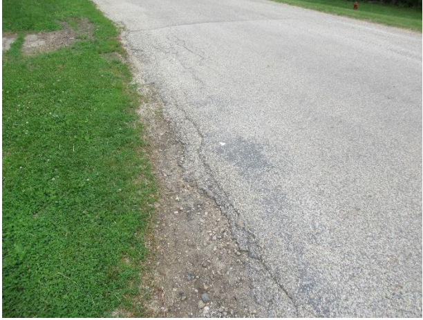
Edge cracks at clubhouse parking area driveway
