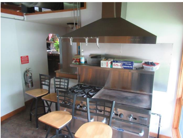
Clubhouse kitchen components
