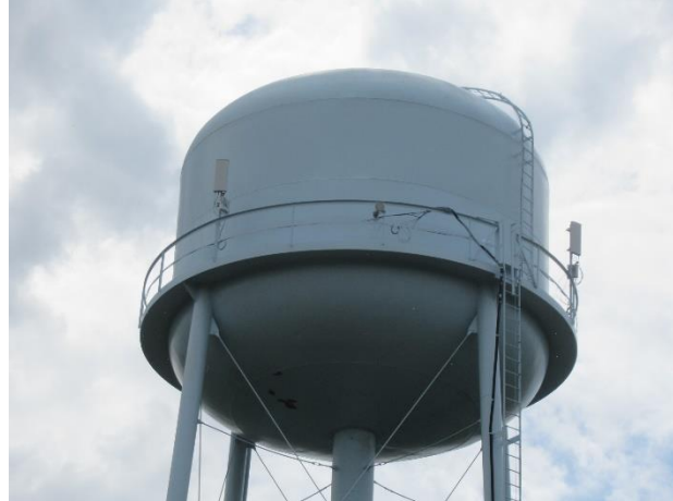
Close-up view of water storage tank
