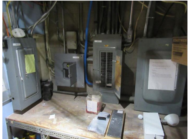
Clubhouse electrical panels
