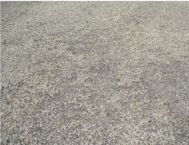
Pavement deterioration at beach parking area
