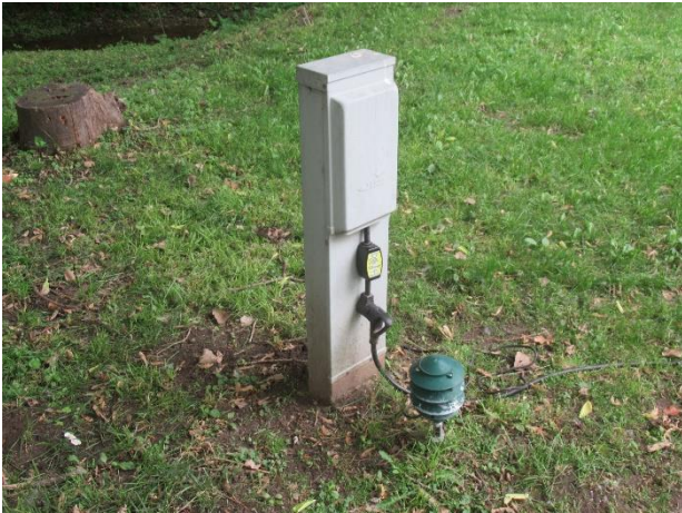
Campground power pedestal
