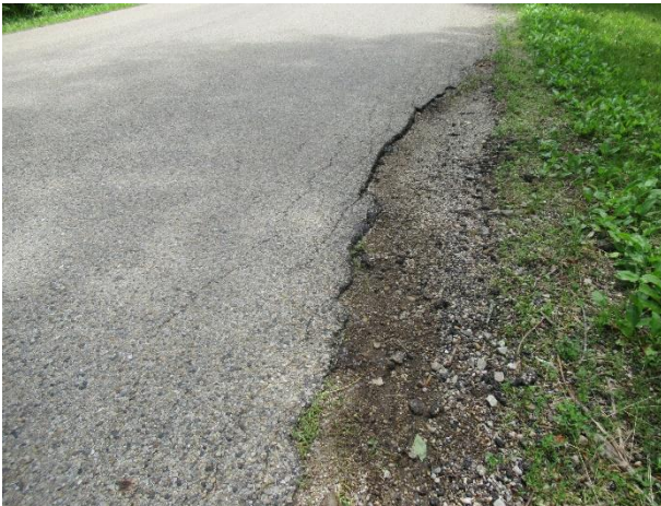
Street edge deterioration
