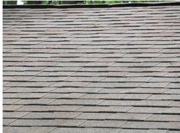
Minor wear and granule loss visible at Snack Shack roof
