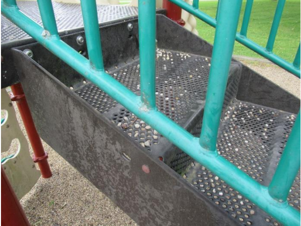
Playset finish deterioration
