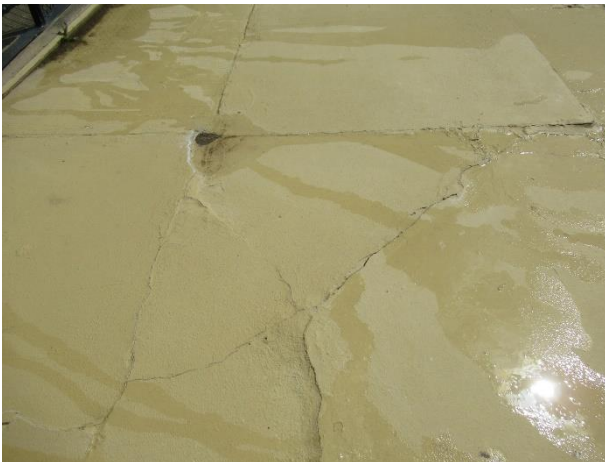
Cracks and settlement
