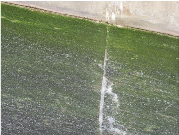
Deterioration at base concrete isolated to control joint areas
