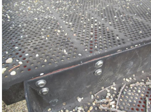
Playset platform deterioration
