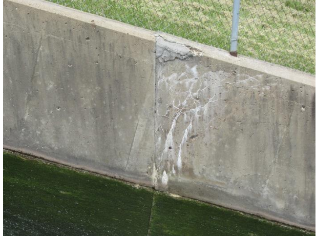
Deterioration and previous repairs visible at spillway walls
