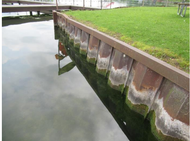
Deflection and deterioration at beach bulkhead
