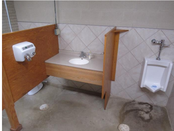
Snack Shack rest room fixtures and partitions
