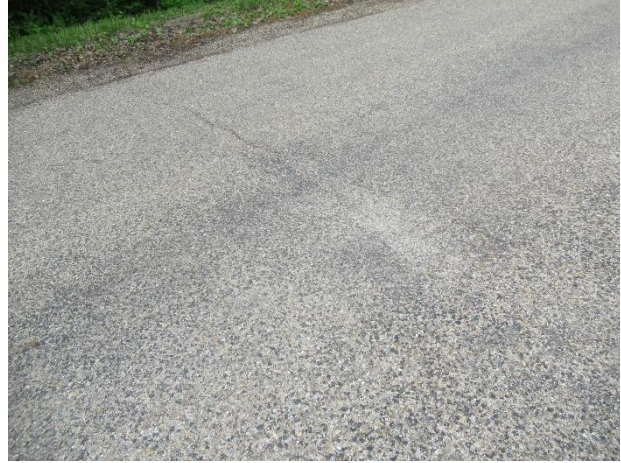
Isolated instance of significant settlement at private street pavement
