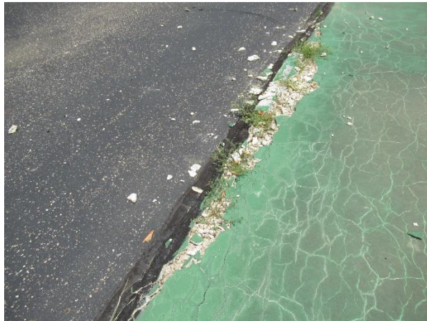
Excessive asphalt deterioration
