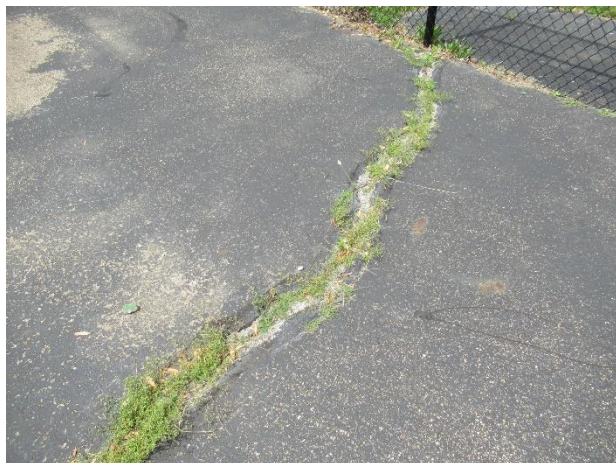
Large cracks found throughout tennis court
