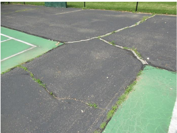
Large cracks found throughout tennis court
