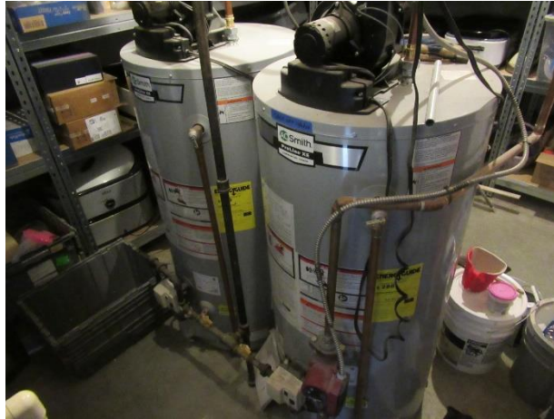
Clubhouse water heaters
