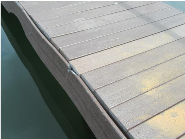
Isolated damage and repair at beach dock
