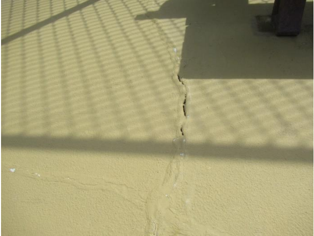
Recurrence of crack at repaired area
