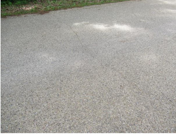
Transverse crack and settlement at private street
