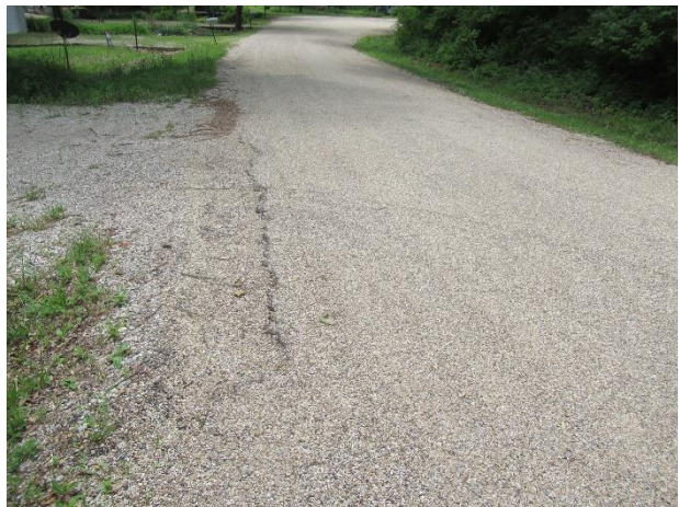
Private street edge raveling at intersection with driveway
