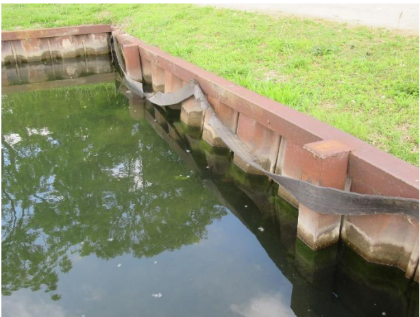
Deflection at clubhouse dock area bulkhead
