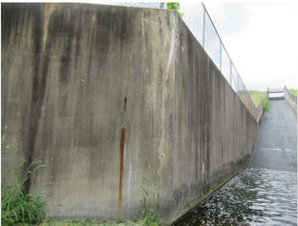
Spillway wall cracks
