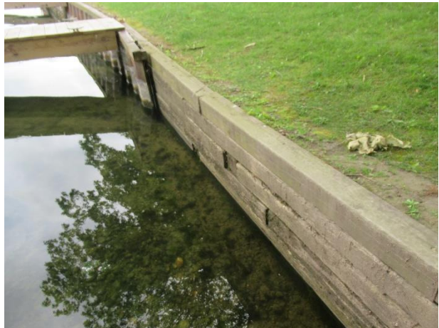
Deflection and deterioration visible throughout wood timber bulkhead area (replace with steel)
