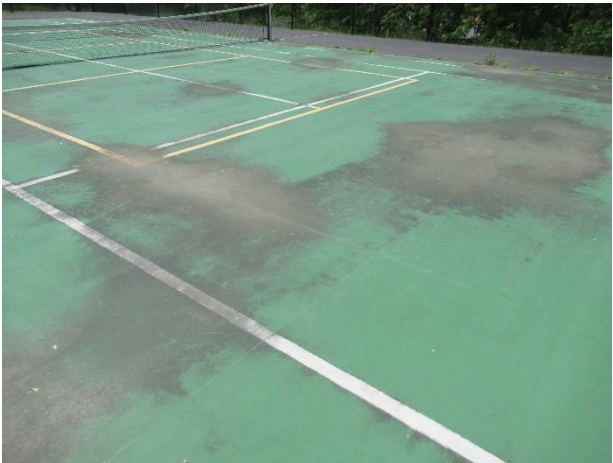
Significant color coat deterioration
