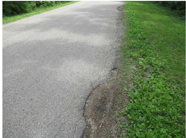
Street edge deterioration
