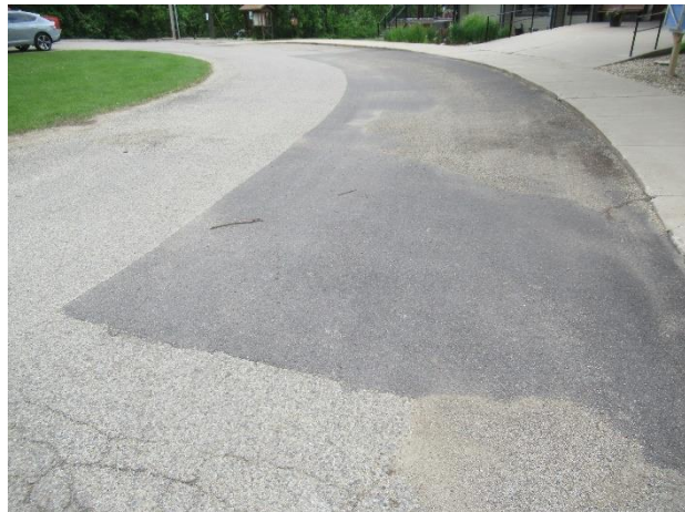
Large pavement patch at clubhouse parking area
